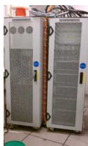
IECO amplifier system installed in the power supply room
