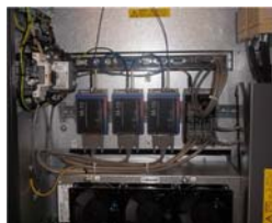
Pyramid controls installed in the amplifier cabinet
